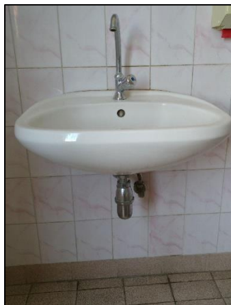
Figure 4 – Washbasin in the toilet of the school
