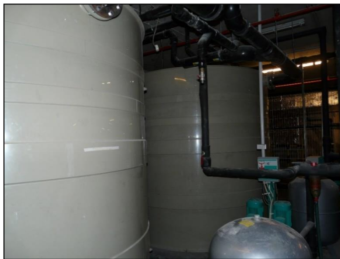
Figure 2 – Greywater-collecting containers, pipe system, filtration device
